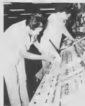
Jose Donata (left) and Maximo Feliciano checking control stations on various panels.
